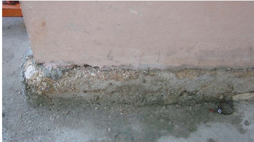
Figure 7. Numerous foundations showed erosion.
