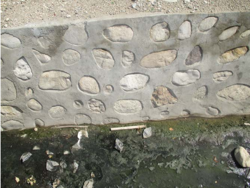
Figure 18. Decorative concrete in an open sewer
