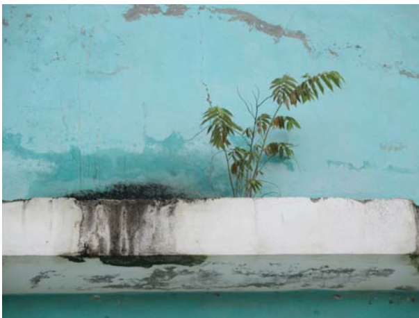
Figure 4. A tree has taken root at the second floor slab which extends out from the wall.
