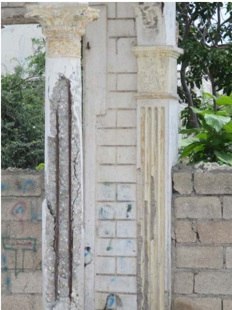
Figure 8. Rebar corrosion caused the face of the column to spall off.
