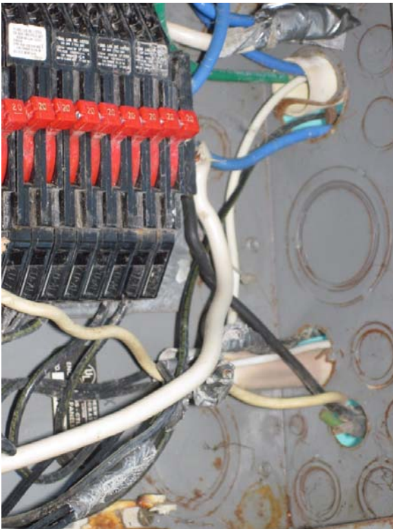
Figure 6. Electrical hookup for a guest house.
