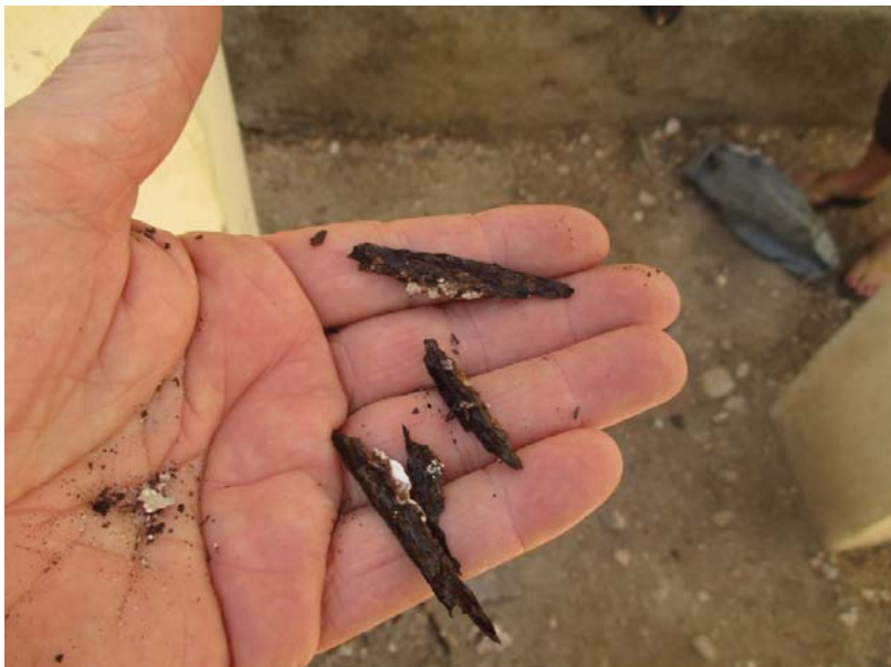
Figure 16. Corroded rebar from overhead water tank.
