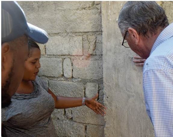
Christie explained to the class why the concrete in the column was eroding.
